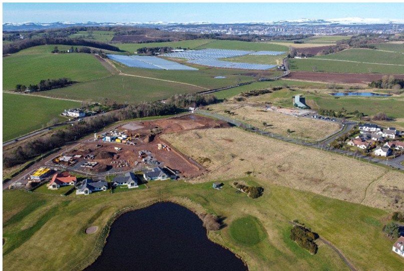
The building site with Dundee and the snow-capped Sidlaws in the background.
